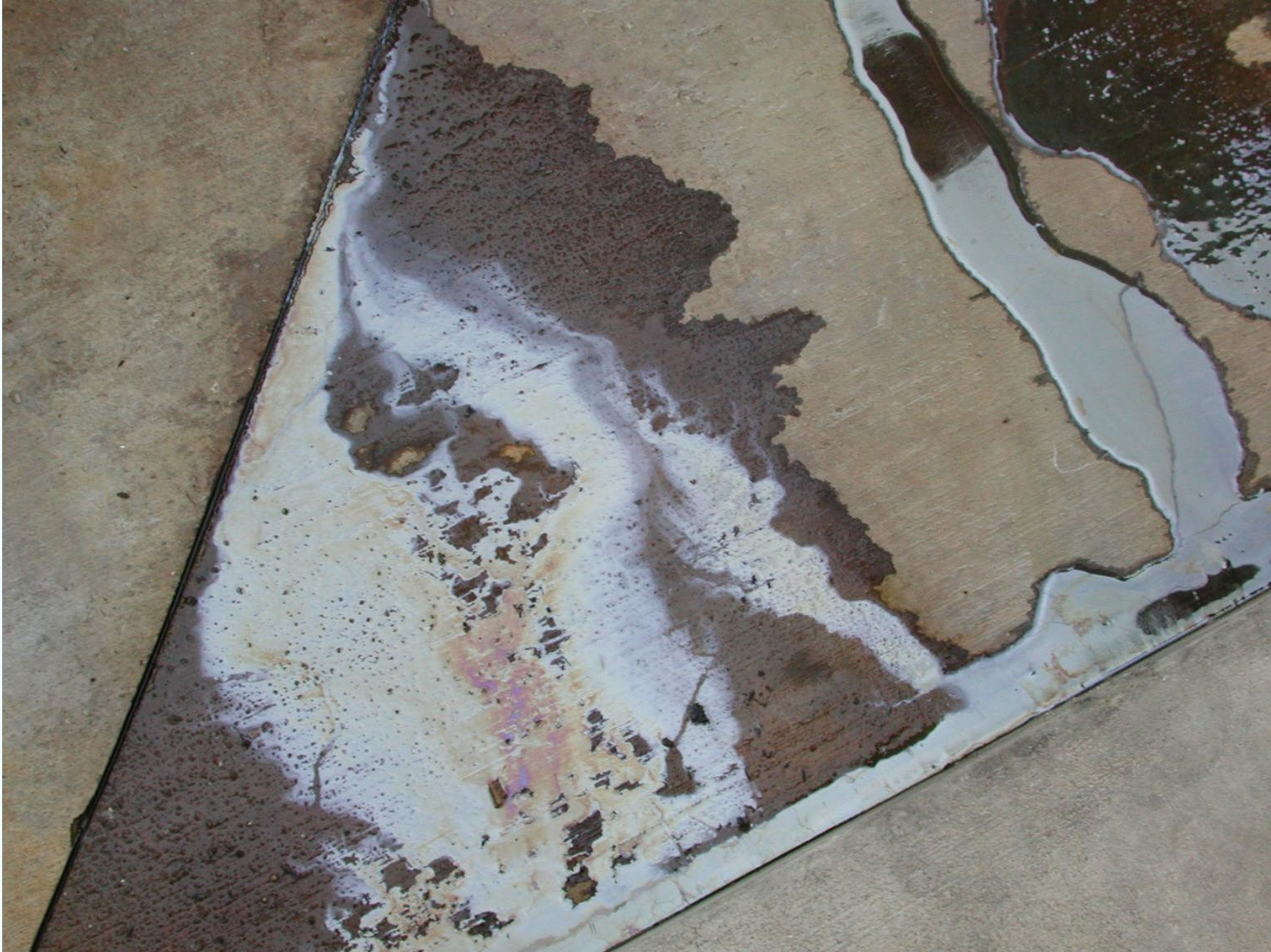
Oily water seeping INTO the containment. Yikes. Not impermeable.
