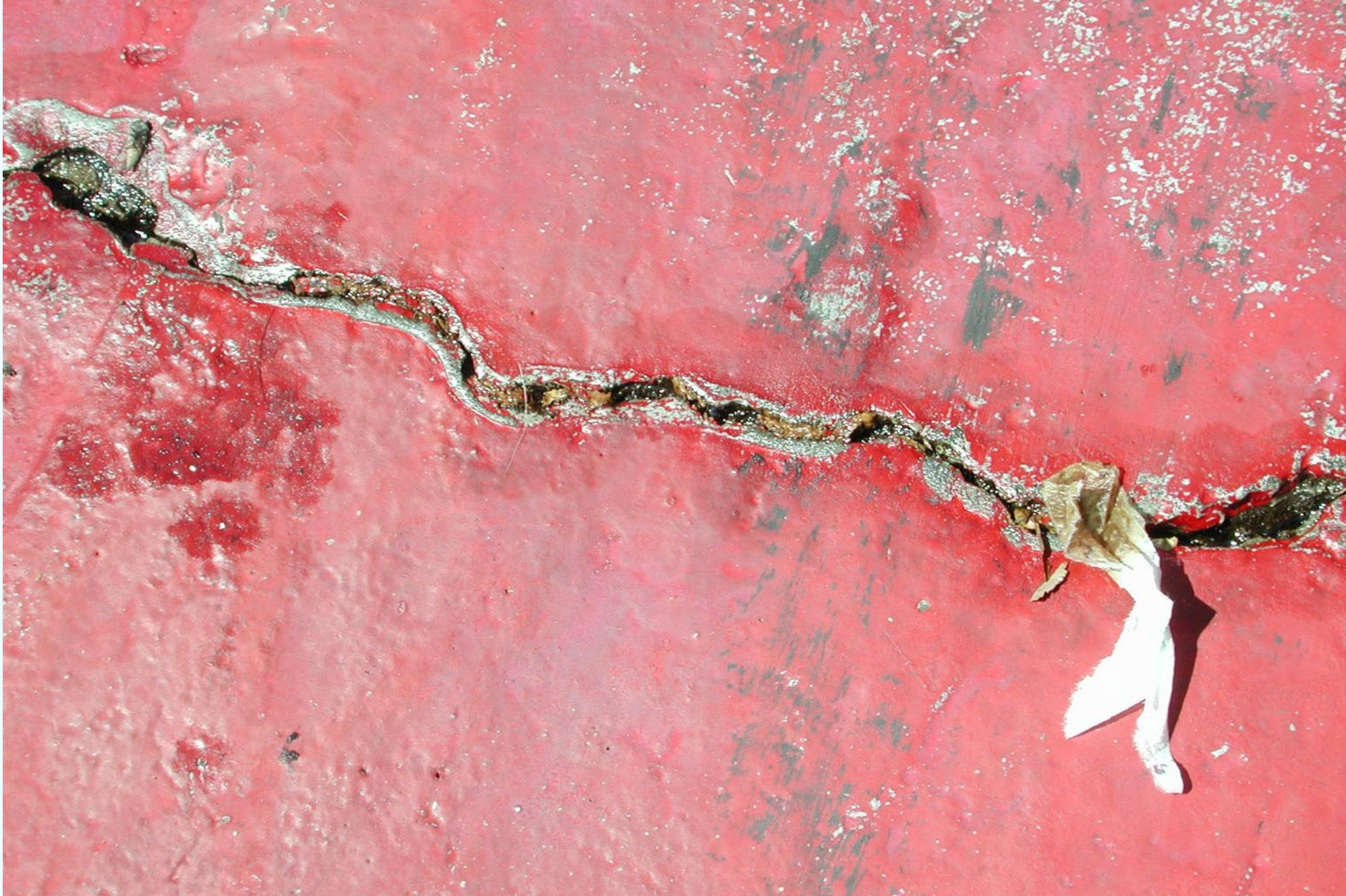
Oily crack in secondary containment (note paper towel absorbing oil).
