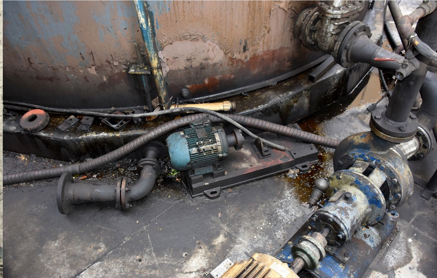
Used oil leaking from a pump and hoses.
