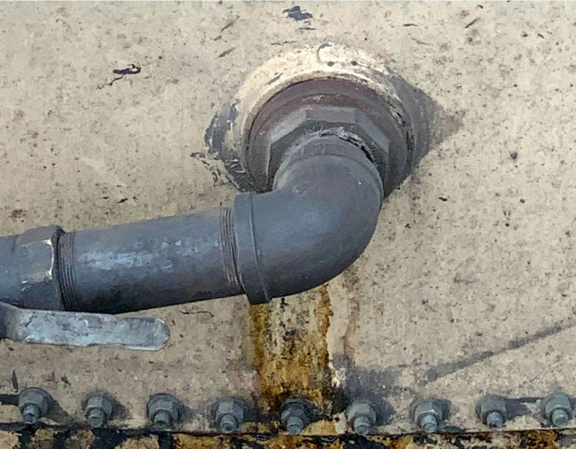
Leak from a pipe seal near bottom of a very large tank. Concerning.
